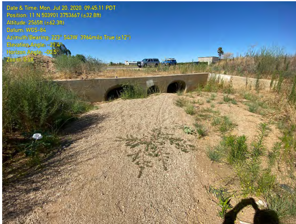
PHOTOGRAPH 7: The culvert at 2 nd Street from the upstream end of Feature C (Potrero Creek).
