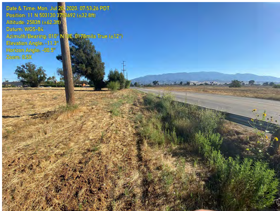
PHOTOGRAPH 4: No roadside drainage was present, or evidence thereof, indicating all flow for Feature A originated from road runoff.
