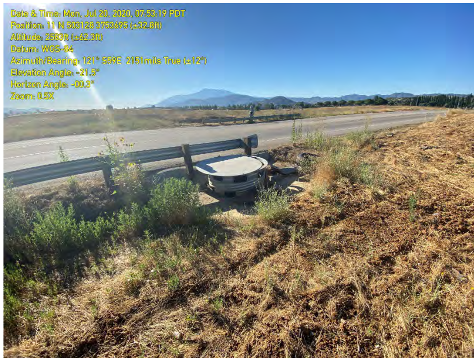
PHOTOGRAPH 3: The westside of Pennsylvania Avenue where storm runoff entered a standpipe connected to the culvert where Feature A began.
